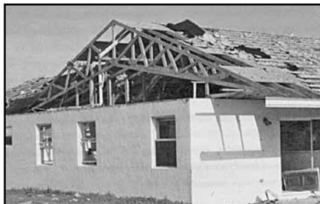
Residential roof gable failure
